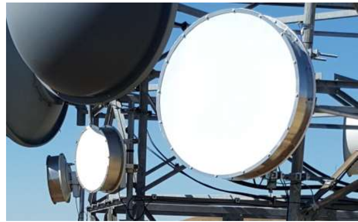
Commercial installation standards, shielding, frequency coordination
